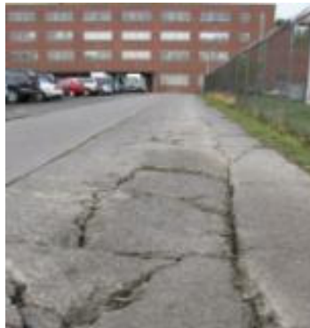
District Wide Road Damage
